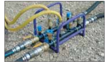
Water distribution manifold.
