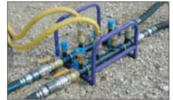
Water distribution manifold.
